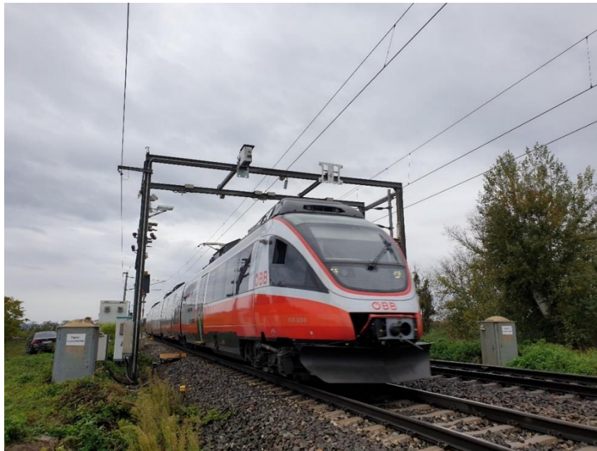
PantoSystem installed on the gantry of ÖBB network in Gramatneusiedl
